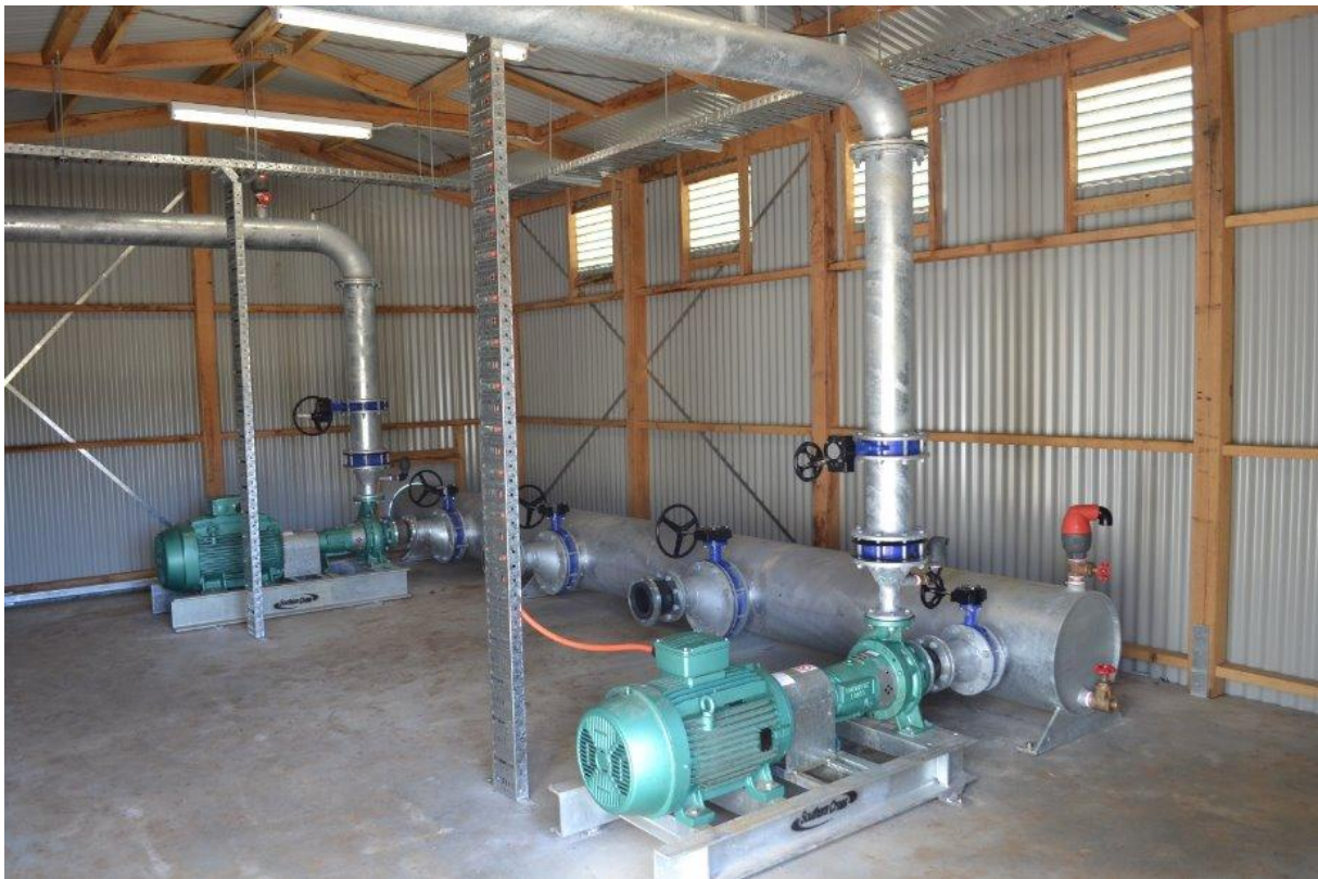
Figure 16: It is important to have a neat and simple design layout for pumping systems for ease of maintenance and safety (Photo: Pinion Advisory)
