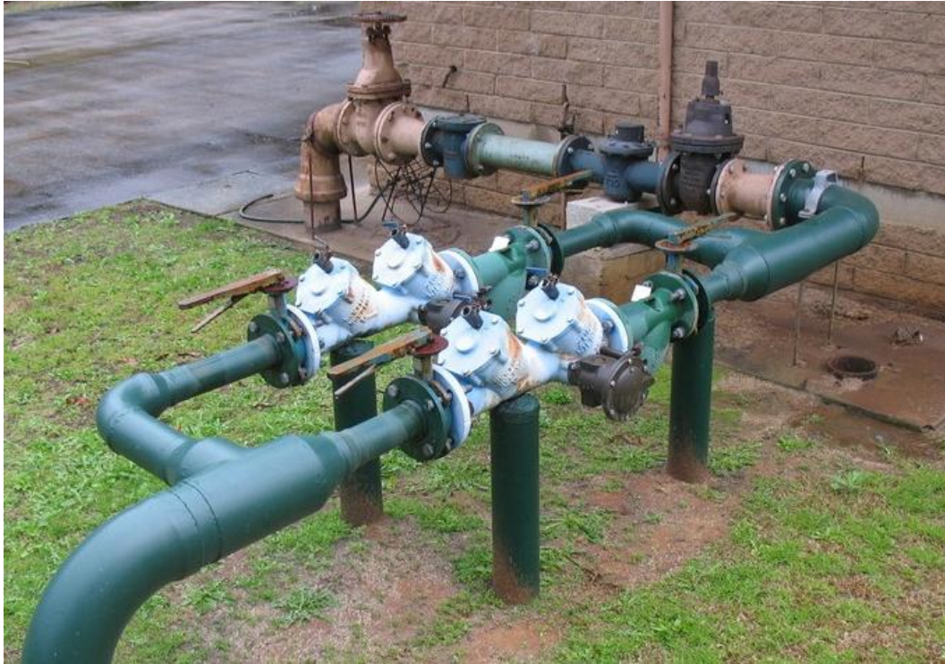
Figure 21: Backflow prevention valve (in light blue) (Photo: (Sydney Water, 2025))
