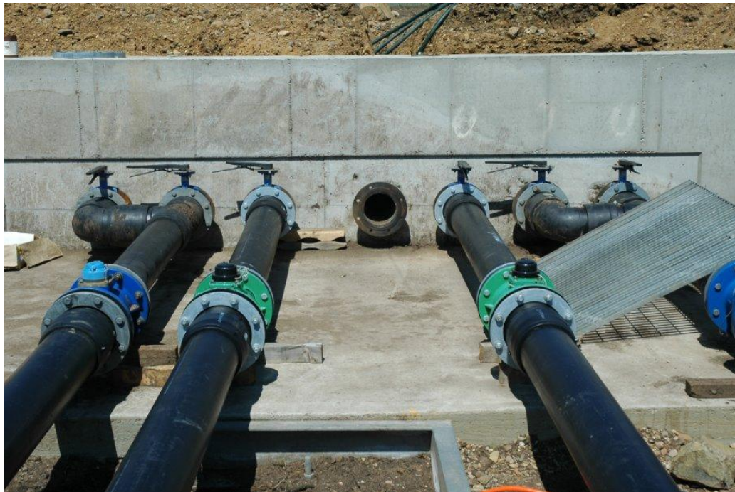
Figure 18: These pipes are made of polyethylene (Photo: Pinion Advisory)
