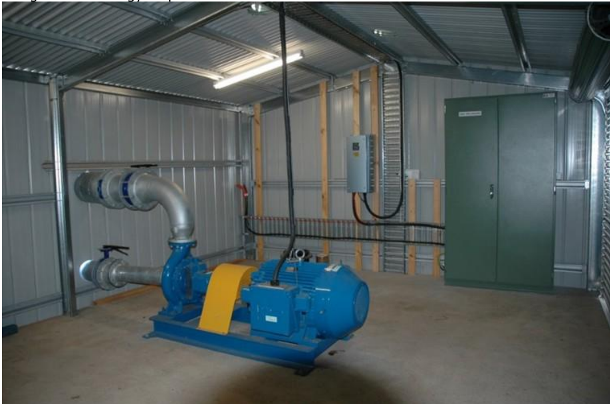
Figure 15: The pump is the critical energy centre of an irrigation system (Photo: Pinion Advisory)
