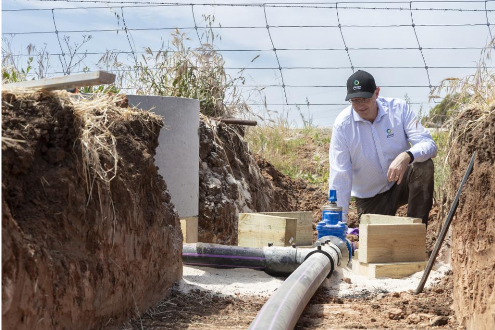
Figure 27: Gate valve. These are often thrust blocked with steel and concrete, as shown here (Photo: Pinion Advisory)
