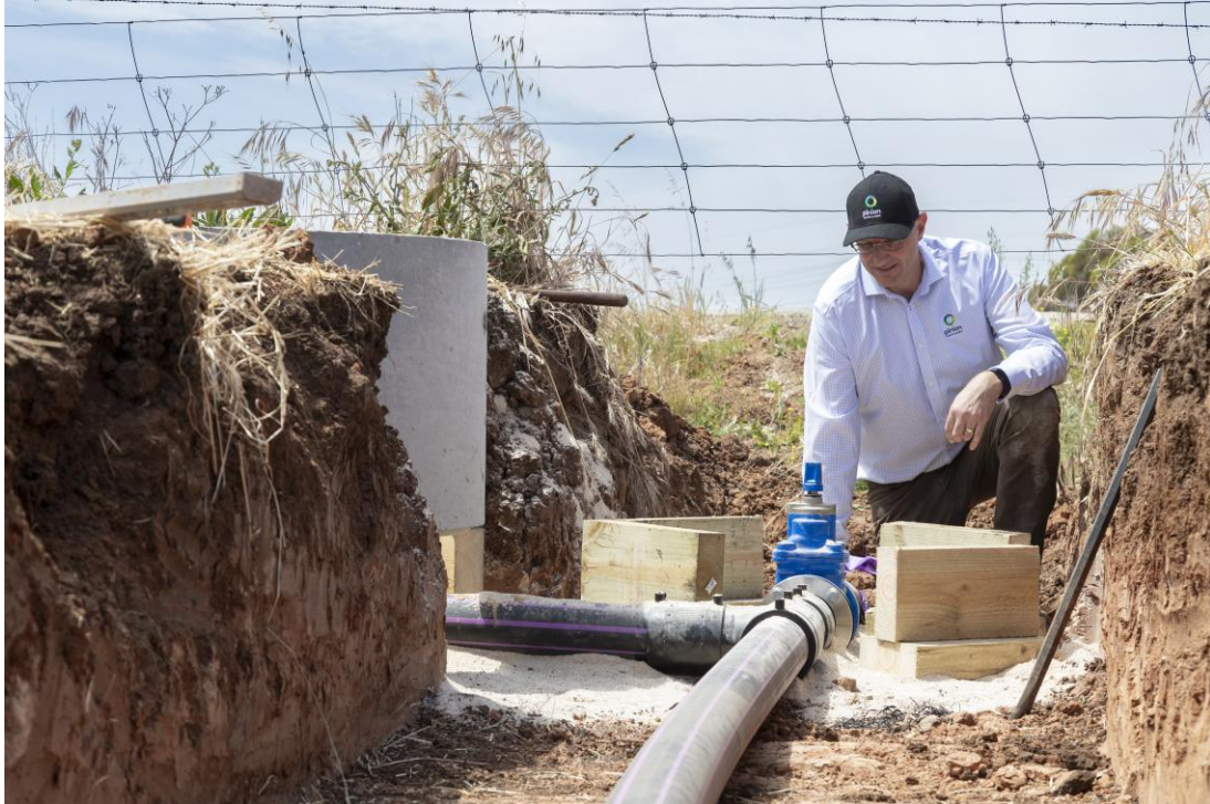
Figure 29: Gate valve. In this example the valve is thrust blocked with concrete (Photo: Pinion Advisory)
