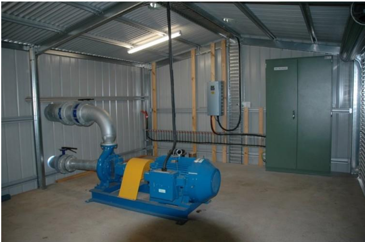
Figure 16: The pump is the critical energy centre of an irrigation system (Photo: Pinion Advisory)
