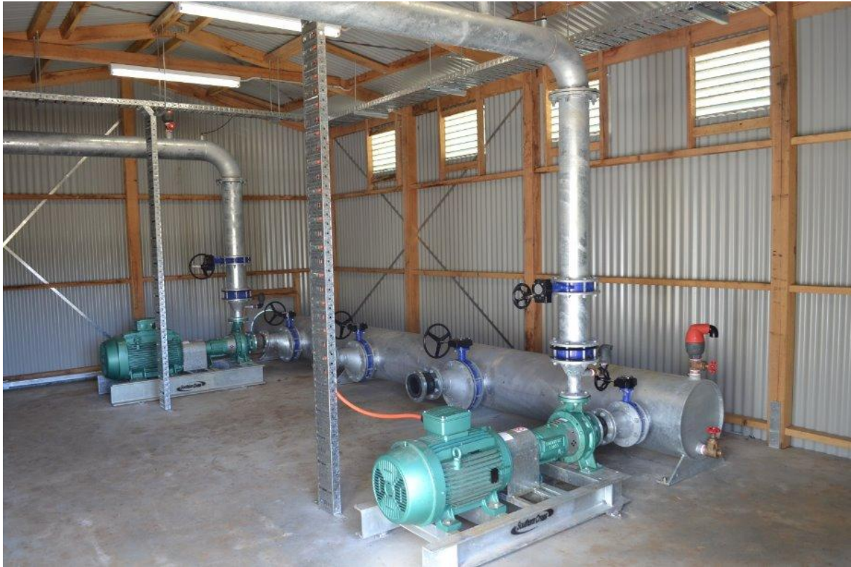
Figure 17: It is important to have a neat and simple design layout for pumping systems for ease of maintenance and safety (Photo: Pinion Advisory)
