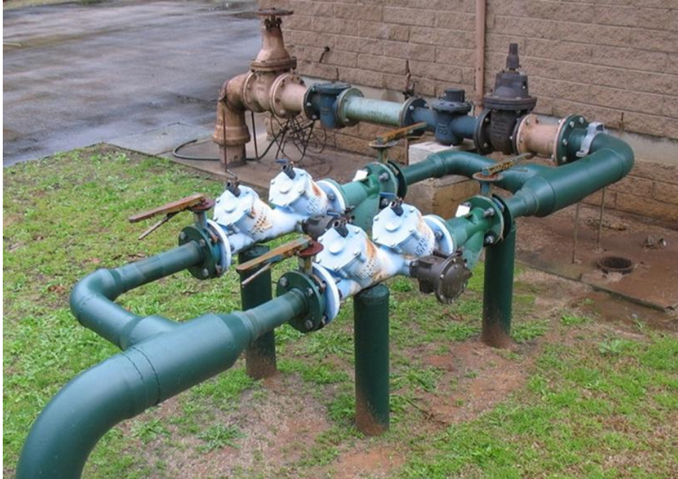
Figure 23: Backflow prevention valve (in light blue) (Photo: (Sydney Water, 2025))
