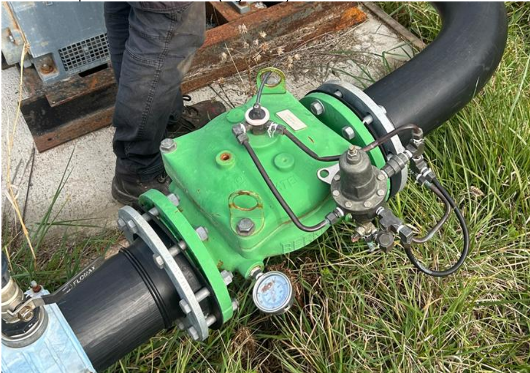
Figure 28: Pressure reducing valve (Photo: Pinion Advisory)
